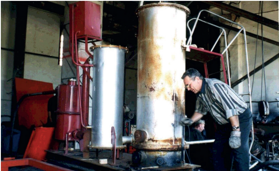
Figure 5. General view of the gas generator GG-30
